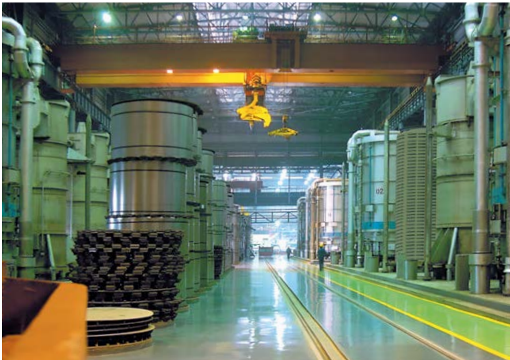
▲ HPH® Bell-type Annealing Furnace Plant for cold rolled steel strip
