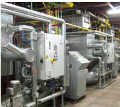
▲ LOI developed Bypass cooling system featuring dual cooler installed in the basement
